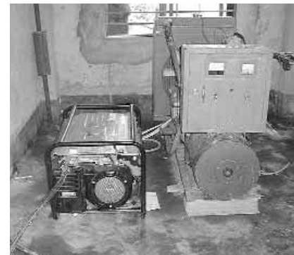
Figure 3.2 Biogas electricity generator at Faridpur Muslim Mission
